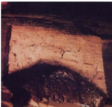
Figure 18. The burn at the tie beam of a truss in the Fencing hall of Fortezza da basso, Florence (Tampone, 1989, cit.).
