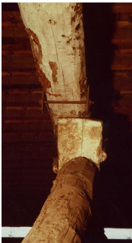
Figure 12. Makeshift assembly, with considerable eccentricity, of a post to the rafter of a truss. The post is deformed (from Tampone, Atlas, 2016, cit.).
