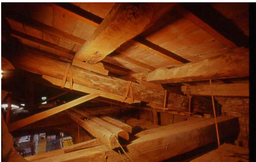
Figure 6. The last strengthening work, composed by an additional stiffening bracket, fixed with iron ties, and by a new strut, was not sufficient to prevent further deformation of the rafter and of the new strut of this truss (Tesi, Tampone, Martini, 1989, cit.). Note the cut made in the bracket to accommodate the end of the strut.
