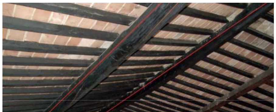
Figure 3. Deflection of a member of a simple roof carpentry, Certaldo.
