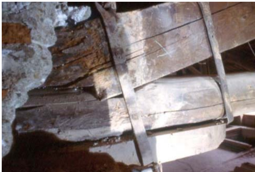
Figure 17. Sliding of the rafter due to rupture of the heel of the tie beam of a truss. The size of the sliding is evident in the picture (18 cm circa). The two collar ties are not correctly placed and do not work efficaciously (from Tampone, Atlas, 2016).
