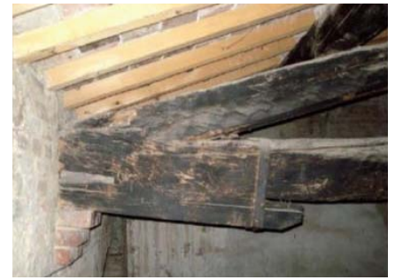
Figure 9. Node of the truss of the Ceraldo Palace of the Vicars roof showing severe failure.
