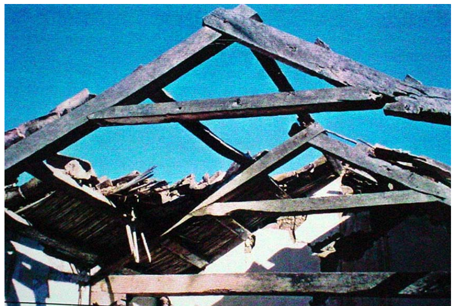
Figure 11. Rupture of a rafter in the joint with the strut due to the hollow made in the member (from Tampone, Atlas, 2016, cit.).
