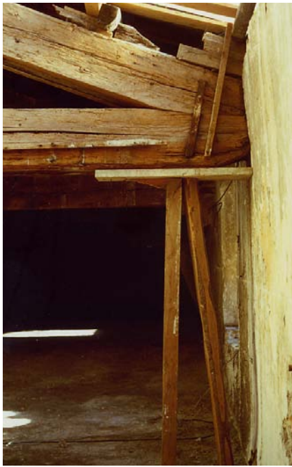
Figure 8. Effects of combined situation of short rafter of a truss and fungal attack of the node. Note the deformation of the tie (Tampone, Atlas, 2016, cit.).
