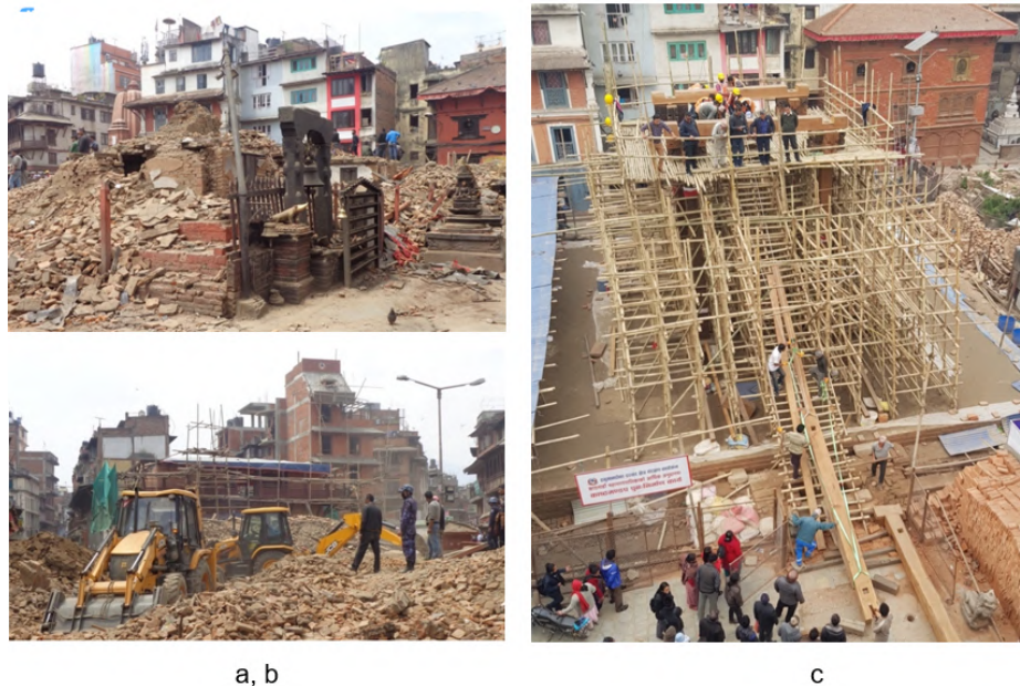
Figure 1: View, the collapsed structure, reconstruction using bamboo scaffolds (Photo courtesy: Kai Weise)
