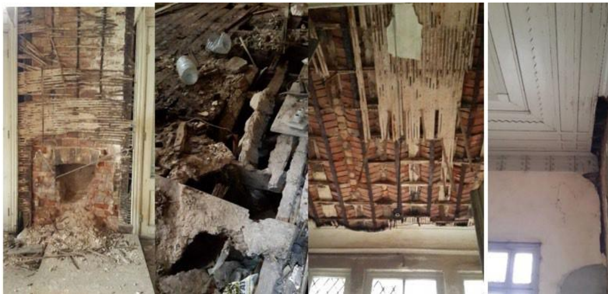
Figure 20: Damage to the masonry parts and floors – 2019.
