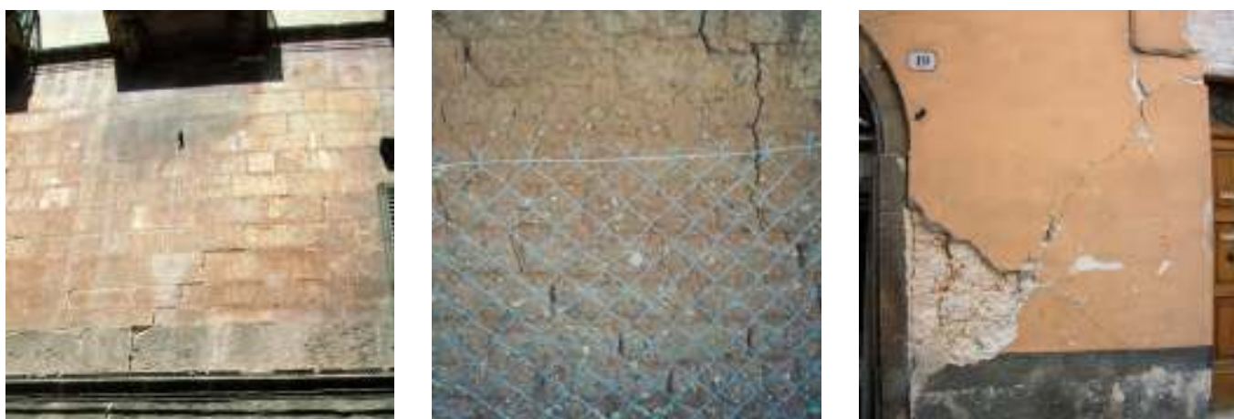
Figure 14. Morphology of shear cracks in 14a. Stone masonry, 14b. Earth masonry, and 14c. Masonry made with small size stones and thick mortar joints.
