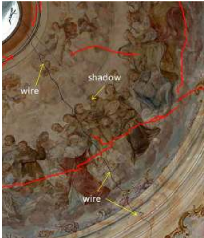
Figure 18. St. Anna's church, mapped real cracks and a crack imitation by a wire, (courtesy of Katarzyna Górecka, Academy of Fine Arts in Warsaw, Poland).
