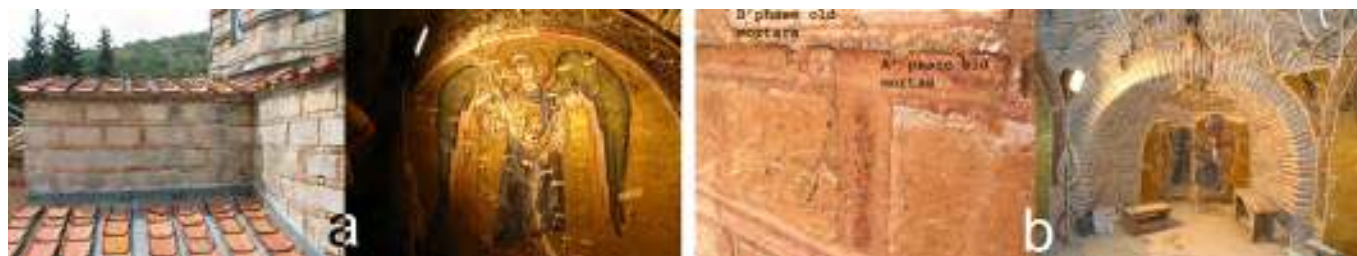
Figure 26a. North external façade of the East arm of the cross bearing old byzantine mortars (left) and the heavily damaged mosaic in its internal façade (right). 26b. External old mortars of 1st and 2nd construction phase (left) and internal precious mosaics, which had to be preserved in situ (right) adapted from [9] © Hellenic Ministry of Culture.
