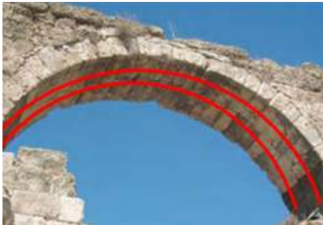
Figure 2. Longitudinal cracks along the arch.
