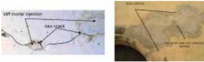
Figures 8. Cracked historical masonry after improper repair using stiff cement mortar.
