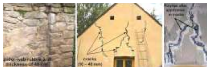
Figures 15. Cracks of masonry family building, constructed from spider-web rubble walls of poor quality, repaired by polyurethane PM flexible joint.
