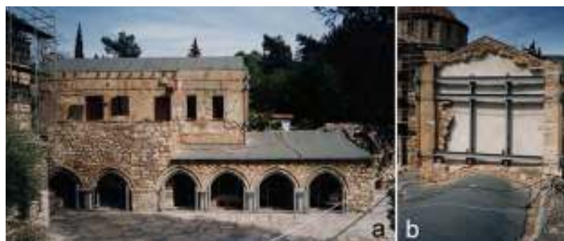
Figure 7a. West façade of the Eastern range of cells and 7b. emergency measures to the collapsed south wall of first floor [8] © Hellenic Ministry of Culture.
