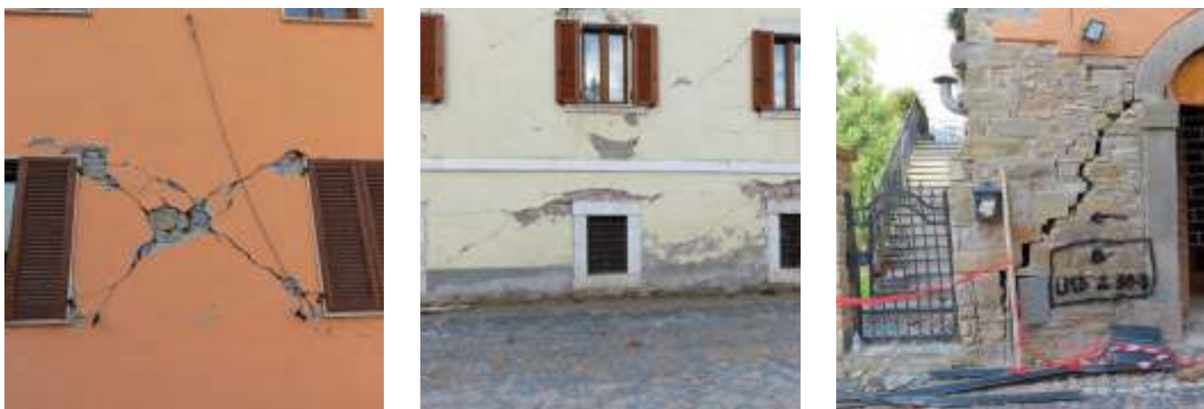
Figures 13. Typical damage due to in-plane shear.
