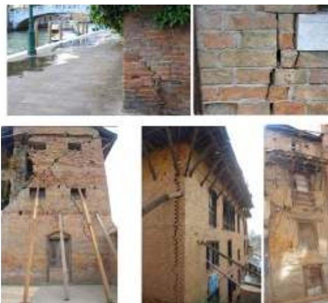
Figures 7. Cracked historical masonry structures with not stable foundation (Venice) and located in seismic areas (Nepal).
