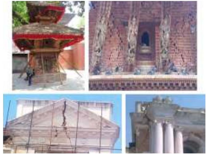
Figures 3. Damaged heritage structures in Kathmandu (Nepal), vulnerable to strong aftershocks.
