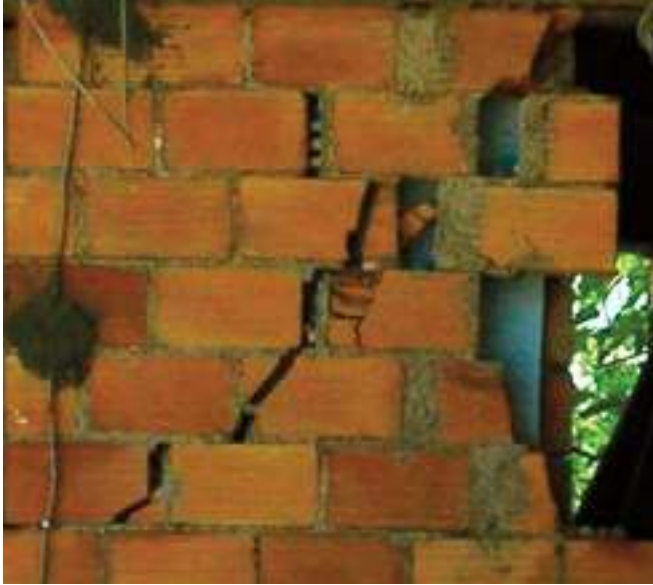
Figure 17. Failure of blocks in various locations along shear cracks.
