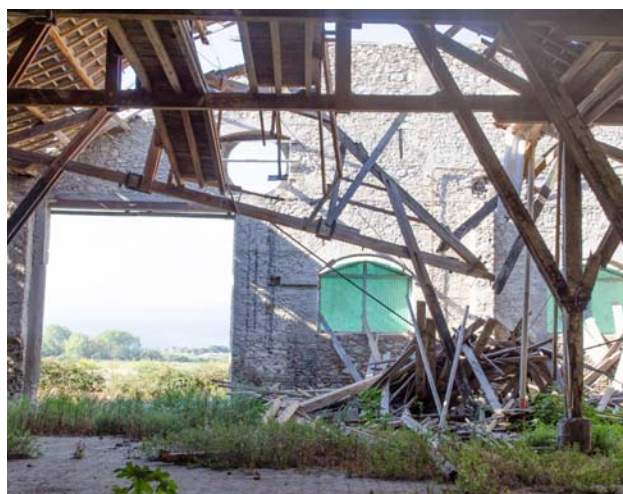
Collapsed trusses in the warehouses (2013 © Micco F. I.).
