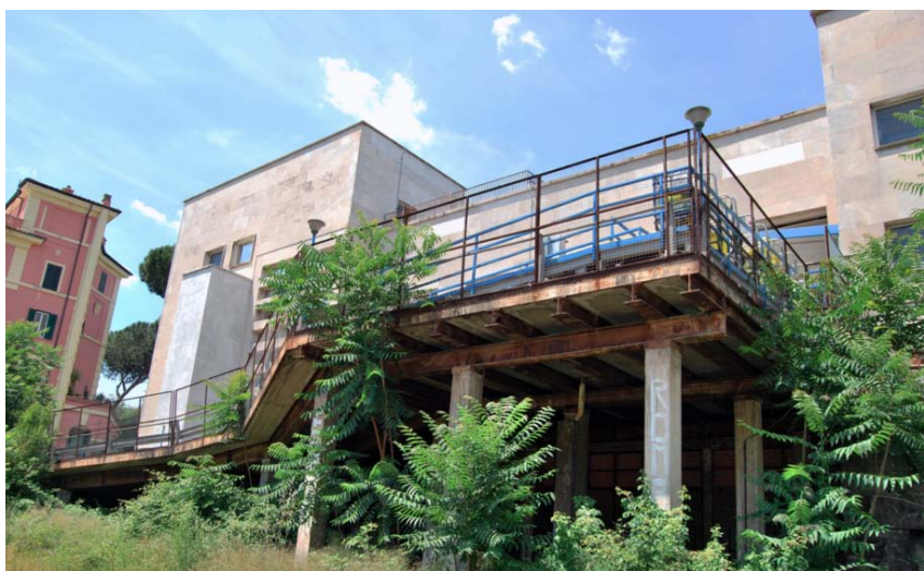
The disfiguring car ramp in steel and reinforced concrete built over the swimming pools façade in the 1970s.
