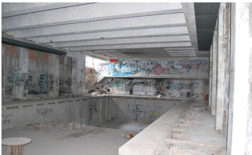
The indoor swimming pool, 2014. The cladding of the walls and the covering of the basin are defaced with paint spray; the flooring is heavily degraded; many windows are walled-up.
